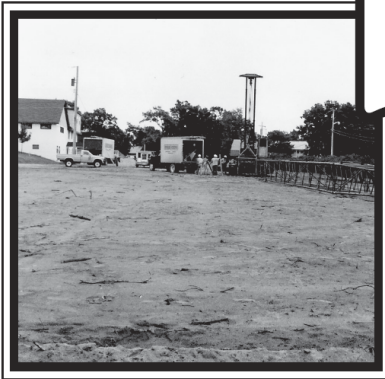
The original parking lot was installed on Wednesday, June 27, 1984 by H.L. Johnson Companies at a cost of $10,100.
